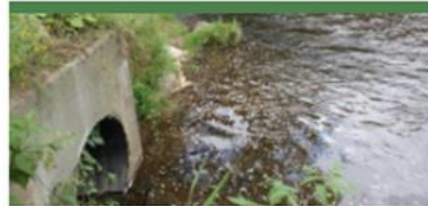
Combined Sewer Overflow
